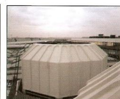
Large evaporative cooling tower
