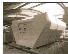
Large packaged chiller
