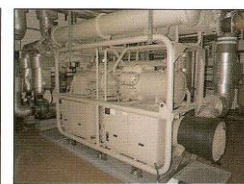
Large water cooled chiller in a plant room
